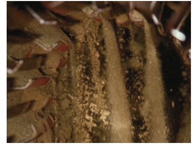
Rotary dryer flights during operating conditions.
